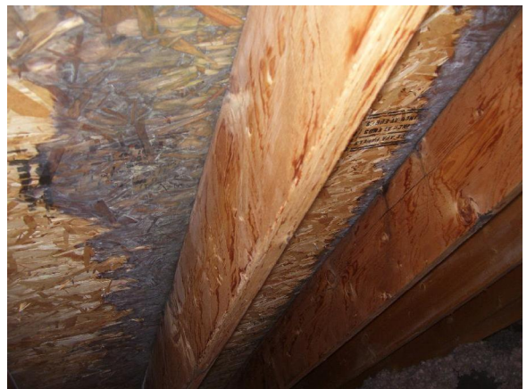
Interior Ventilation & Insulation Mold like substance present in attic
