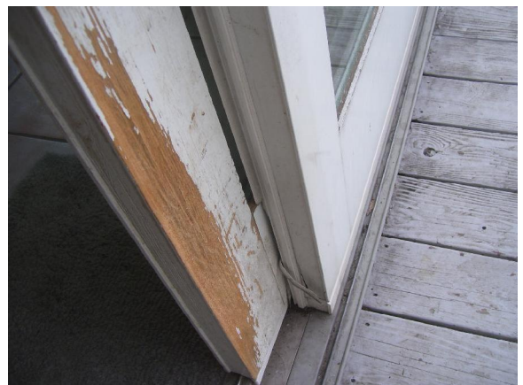
Interior Doors/Windows Deteriorated patio door
