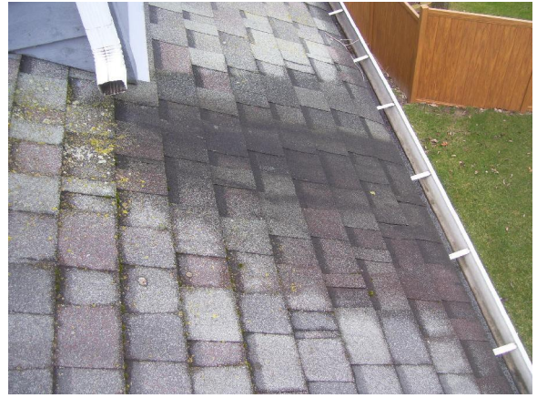
Roof Roof Conditions Accelerated wear due to downspout on north side
