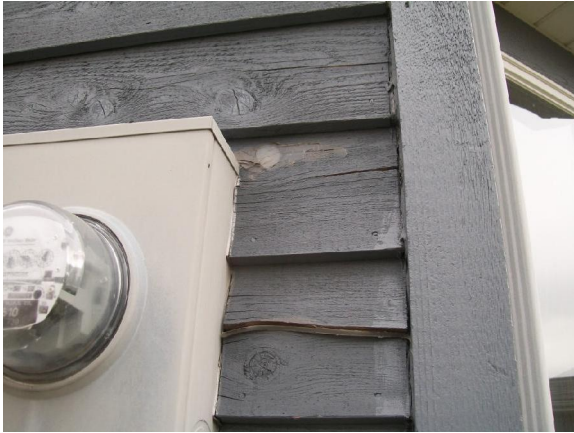
Structure Exterior Walls Deteriorated wood siding
