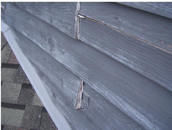
Structure Exterior Walls Deteriorated siding
