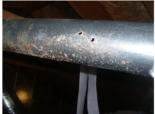
Heating Venting Deteriorated vent in attic
