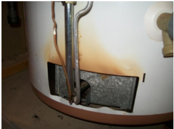
Plumbing Water Heater Condition Backdrafting at water heater in basement
