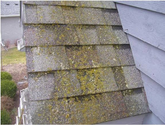
Roof Roof Conditions Moss is present on north side
