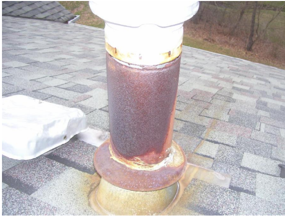
Roof Chimney Deteriorated vent at roof termination
