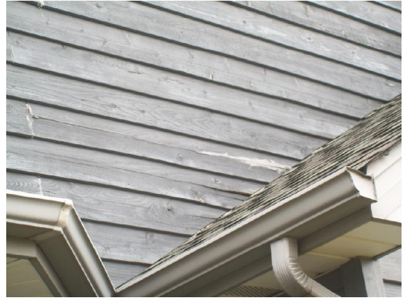
Structure Exterior Walls Deteriorated wood siding
