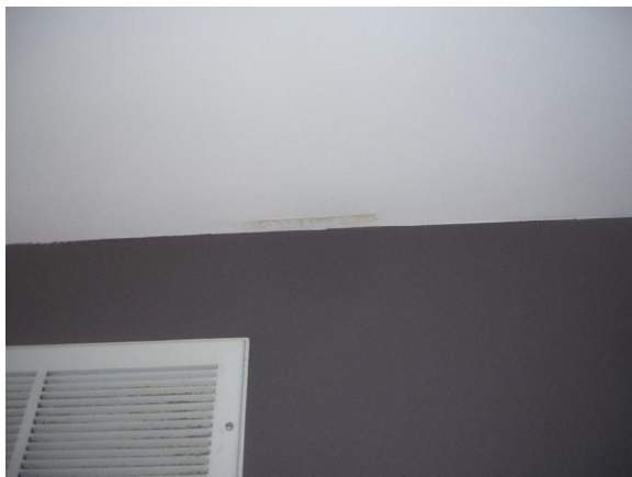
Interior Walls/Ceilings/Floors Stains noted on Master Bedroom ceiling
