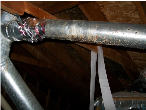
Heating Venting Deteriorated flue pipe in attic
