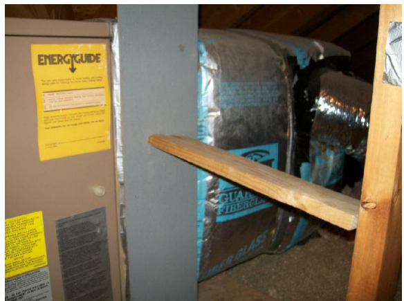
Heating Air Filters Temporary means of sealing off filter
